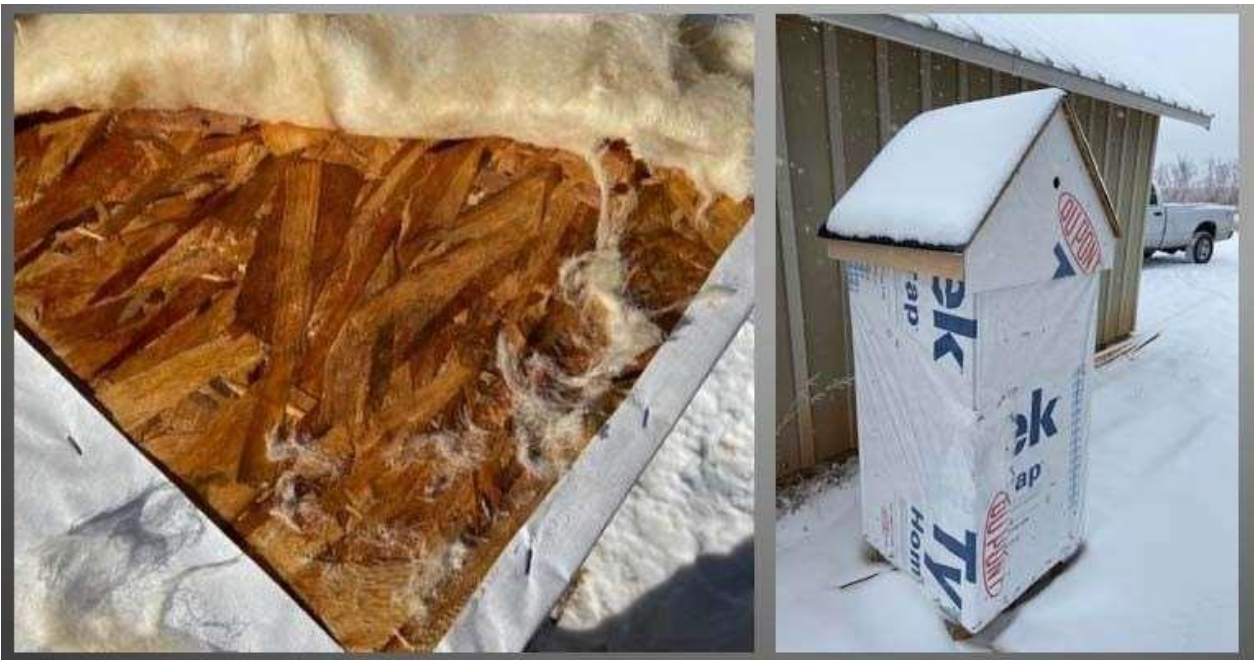
Significant Moisture Condensation at Inside Surface of Exterior Wall Sheathing Test Building Interior at 72 ° F and 42% RH, Exterior 38 ° F and 53% RH Meyers - February 2020 ICC-ES Hearing Testimony
