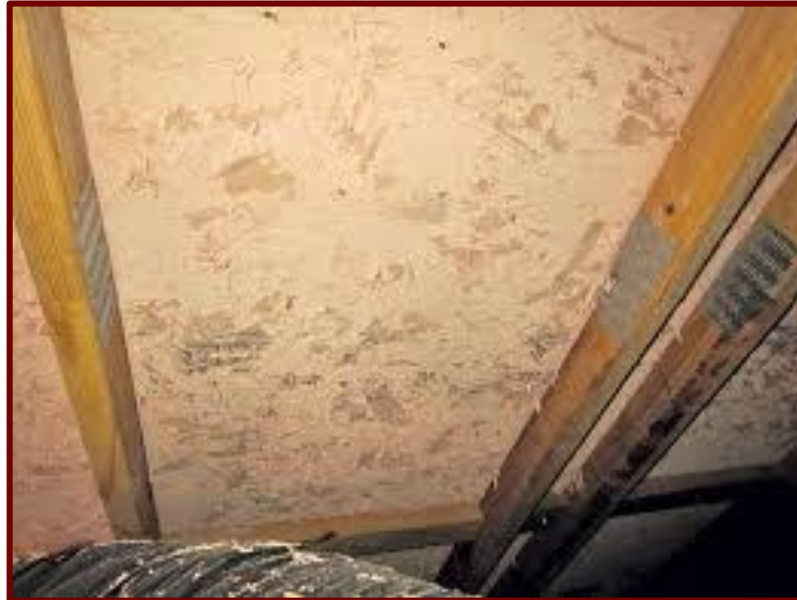
Roof Deck OSB - Intumescent Coating flaking off
