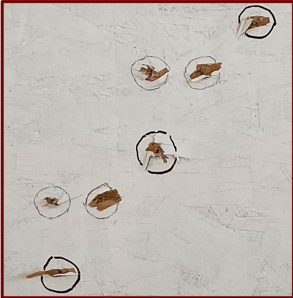
Nail Penetration Delaminated Surface on OSB, Pneumatically Placed Roofing Nails at Industry Standard 90psi
