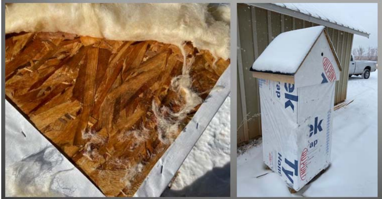
Significant Moisture Condensation at Inside Surface of Exterior Wall Sheathing Test Building Interior at 72°F and 42% RH, Exterior 38°F and 53% RH Meyers - February 2020 ICC-ES Hearing Testimony
