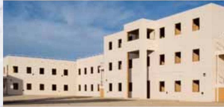
Construction crews install the Ecolite Metal Stud-Framed Lightweight Concrete Wall Panels at the U.S. Army's National Training Center in Fort Irwin, CA.
